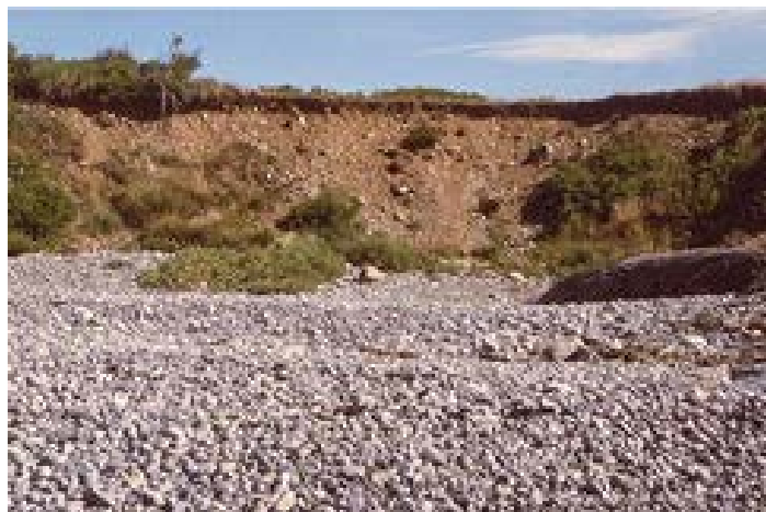
Bluff erosion and gravel beach formation at Fletcher Neck in Biddeford. Maine Geological Survey photo by J. T. Kelley.
